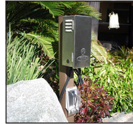
Focus Transformer Mounting
