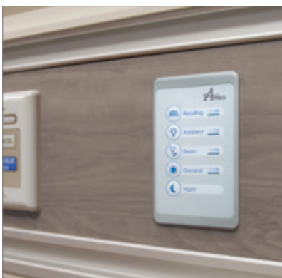
Lights Controlled at Headwall
