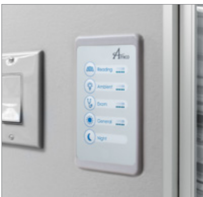
Lights Controlled at Patient Room Door
