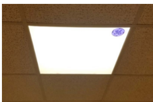
2ftx2ft recessed luminaire
