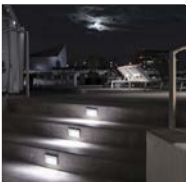
STEP + WALL LIGHTS
